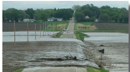
Flooding over County Road D-15 in Ida County.
