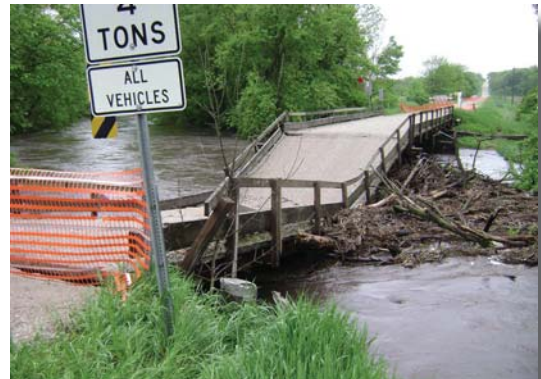
Recent flooding damaged this bridge located in Story County.
