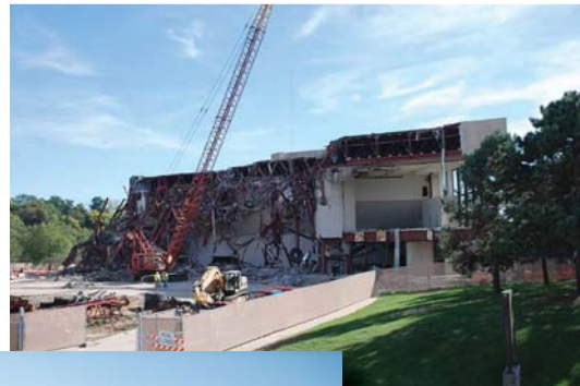
Below: Recovery work on Hancher Auditorium at the University of Iowa, which sustained severe damage during flooding in 2008.
